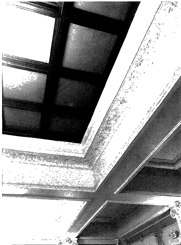
© HDG Special to the Register Jack Hatch says the finished work of the craftsmen is indistinguishable from the original molding in the completed restoration of the ballroom
